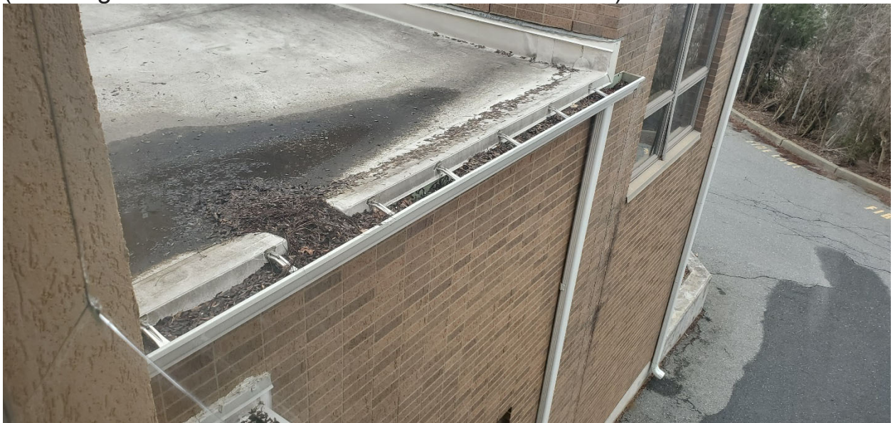
(When gutters are clogged, water builds up on the roof)
