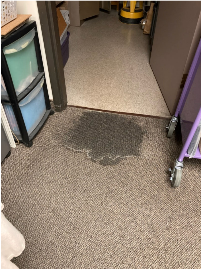
(Mysterious pool of water coming up from the floor in the Circulation Department)
