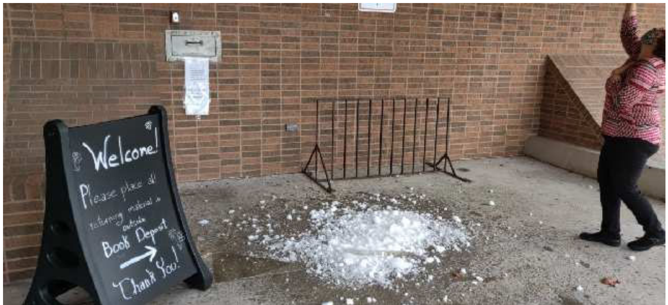
(December 2020: Gina assessing the situation after both skylights crashed down over the entrance to the library following snow and icy conditions)
