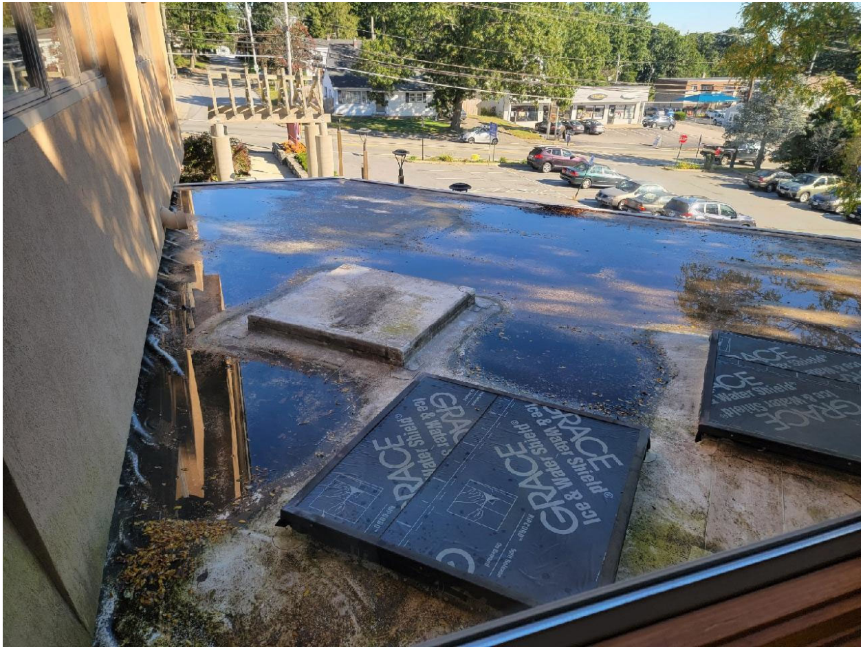
(standing water on the roof above the front entrance)
